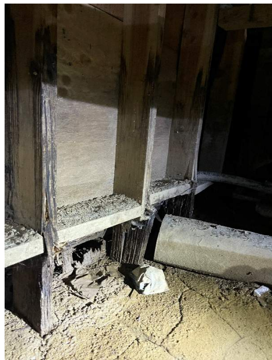
Photo S2- Wood studs and plywood in crawl space under east corridor bearing wall.
