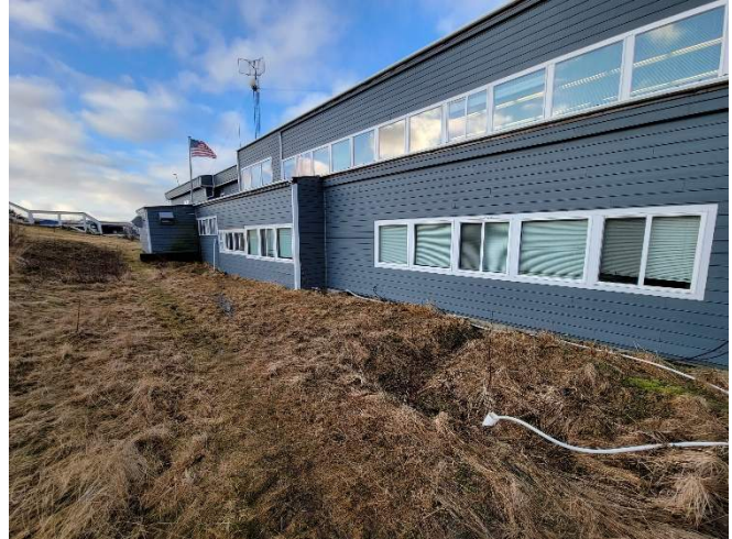
PHOTO OF THE 1975 ADDITION AT THE MAIN LOCATION OF WATER ENTRY INTO THE CRAWL SPACE
