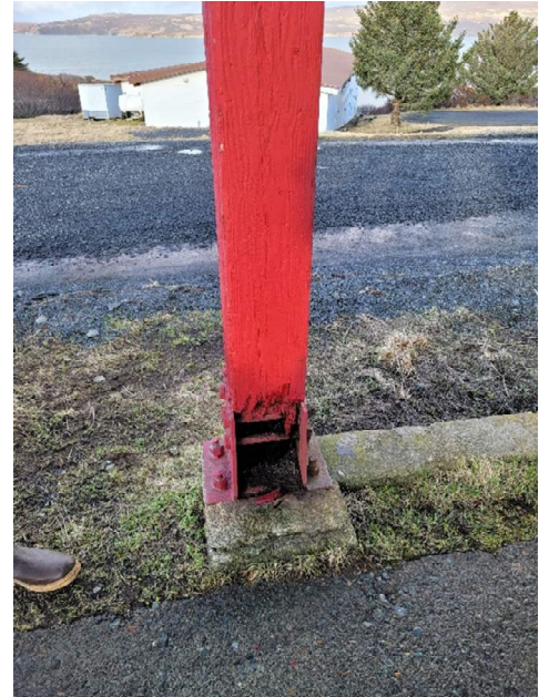
EXTERIOR POST ROT AT THE 1971 BUILDING
