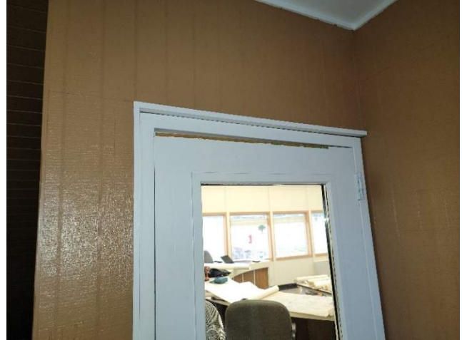
VIEW OF A TYPICAL DOOR AT THE 1975 ADDITION – NOTE THE GAP DUE TO BUILDING SETTLING
