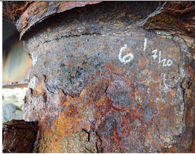
Crack in shoreward-most pier, Pile #6. Approx. 16-inches long on seaward side of pile, below pile-pier cap welded connection.
