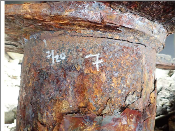
Crack in shoreward-most pier, Pile #7. Approx. 13-inches long on seaward side of pile, below pile-pier cap welded connection.
