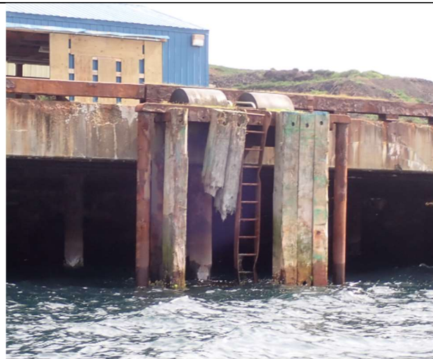
Fender panel #5 is typical, 4 of 8 fender timbers remain. Steel connection brackets exhibit heavy corrosion and impact damage.
