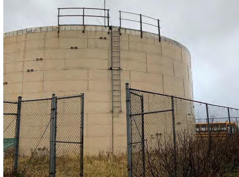
Photo 4. Broken water tank ladder
