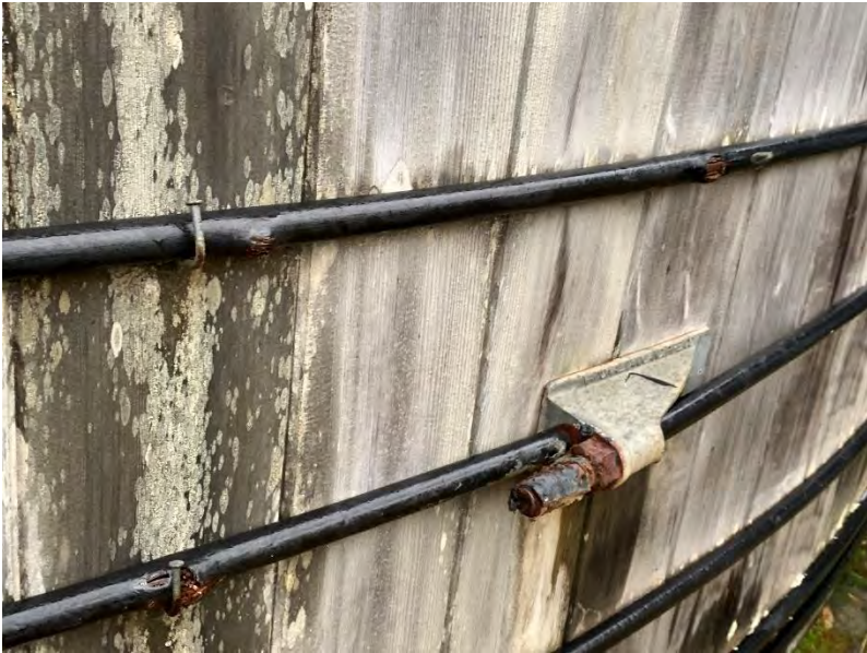
Photo 3. Splitting water tank strap
