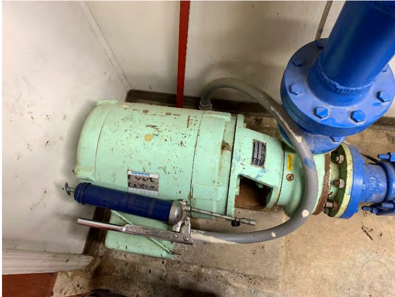
Photo 6. Nonfunctional booster pump at school pump house
