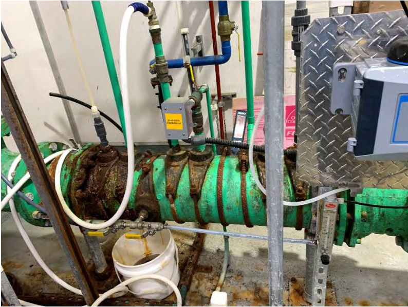
Photo 1: Corroded chlorine injection.
