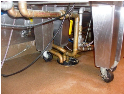
Figure 8: Rotisserie in FSE Without a Grease Interceptor
