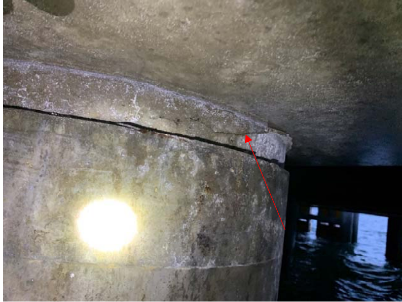
Figure 5: Cracking at Pile B9
