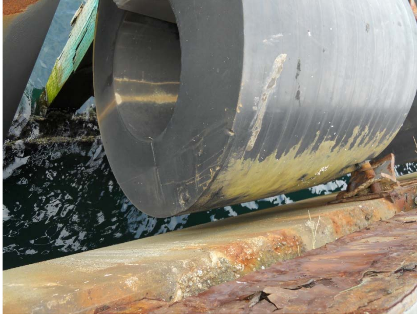
Figure 21: Fender disconnected from dock
