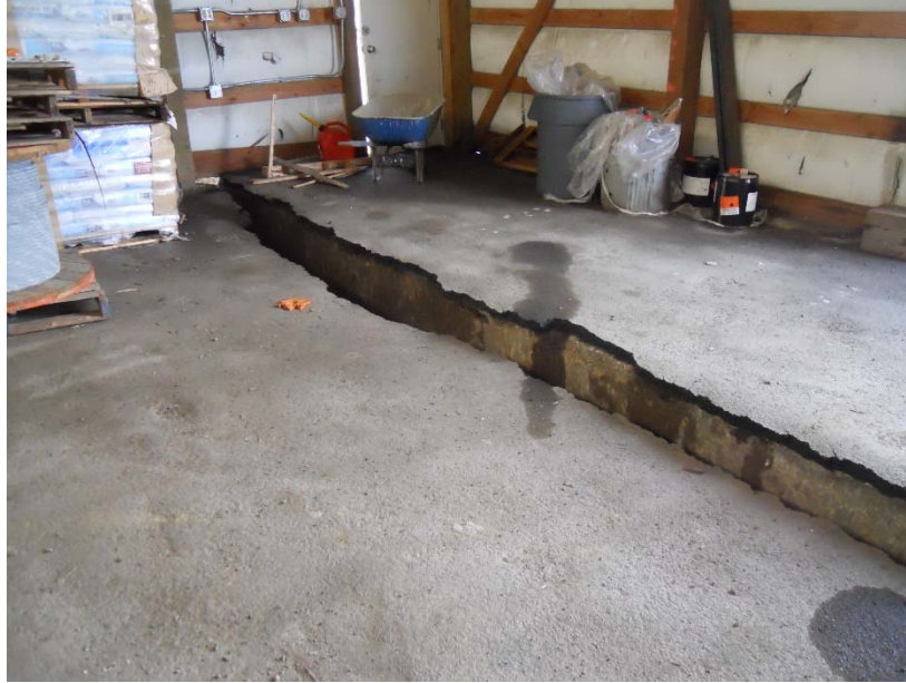
Figure 26: Metal building floor settlement
