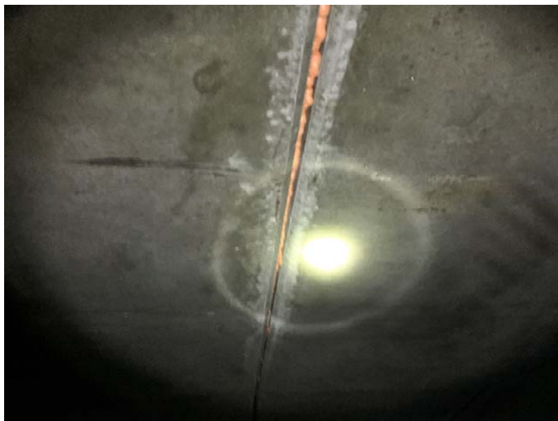
Figure 8: Spray foam on bottom of joint, note salt-water staining adjacent to joint
