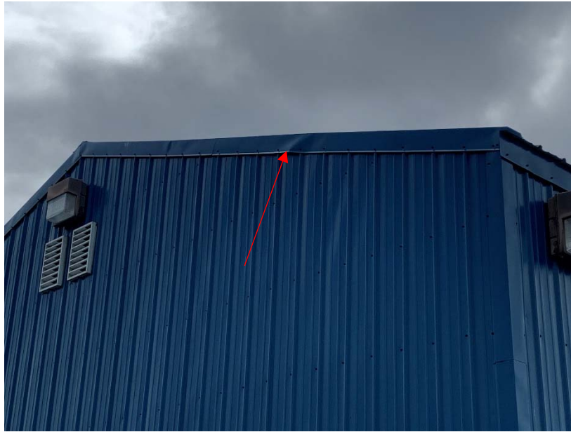
Figure 28: Roofline damage (typ north and south sides, same location)
