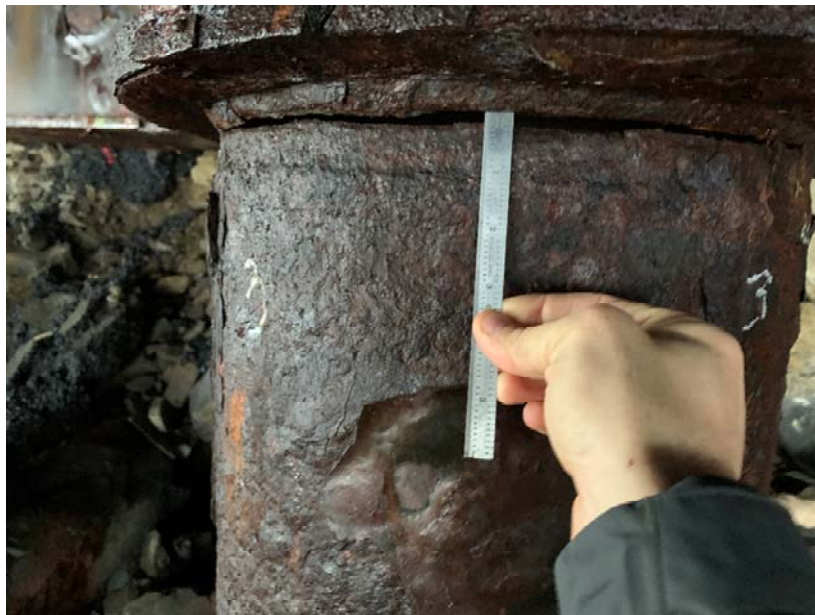
Figure 17: Weld interface crack at Pile A3
