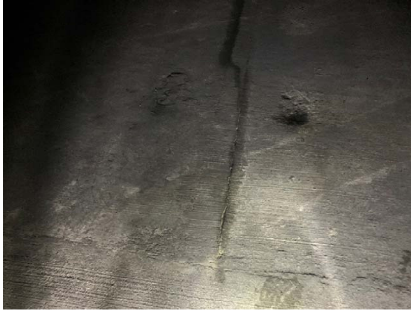
Figure 7: Typical topside grout line cracking
