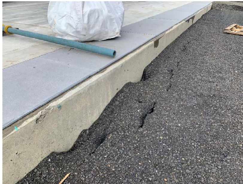
Figure 2: Fill settlement against abutment
