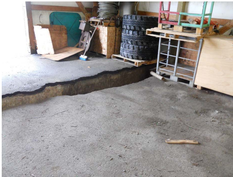
Figure 27: Metal building floor settlement
