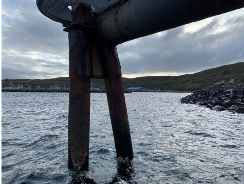
Figure 23: Damaged batter pile
