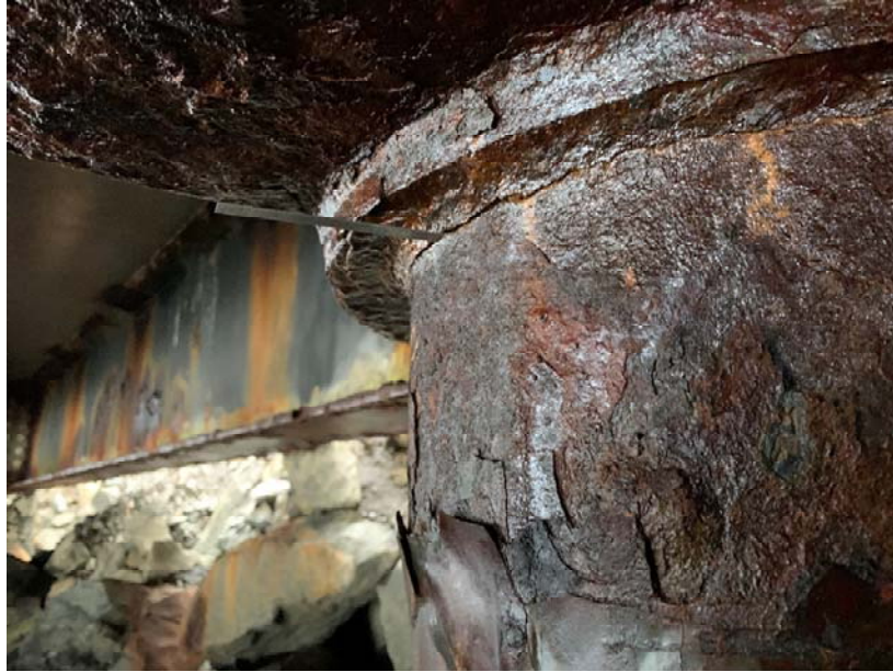
Figure 16: Weld interface crack at Pile A7
