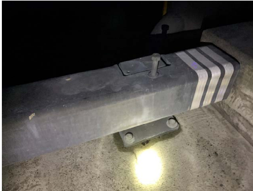
Figure 11: Disengaged bolt in bullrail near gridline D3.5
