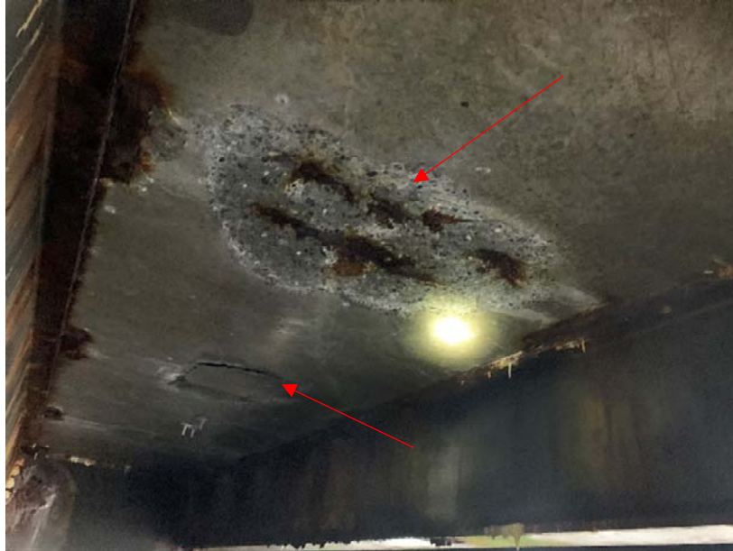
Figure 20: Fully spalled and nearly spalled sections
