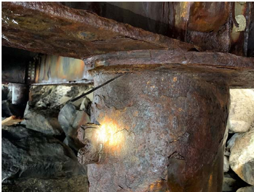
Figure 15: Weld Interface crack at Pile A6
