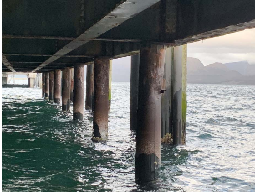
Figure 18: Impact Damage to Pile D3
