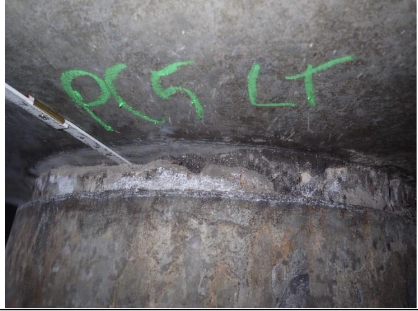
Pile to Pile Cap Interface Spalling
