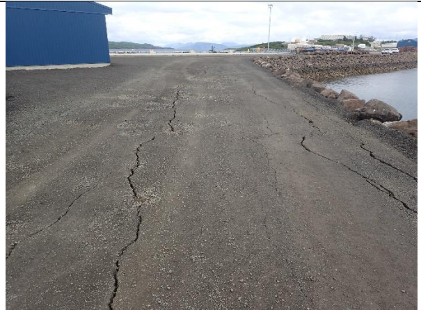
Cracks in Roadway on Breakwater
