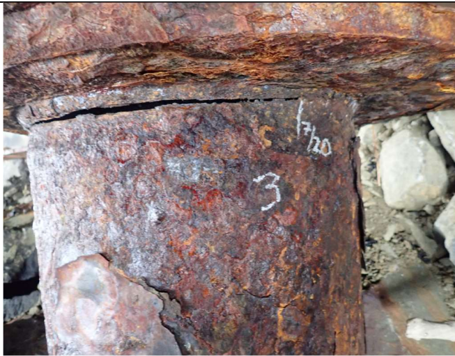
Crack in shoreward-most pier, Pile #3. Approx. 19-inches long on seaward side of pile, below pile-pier cap welded connection.
