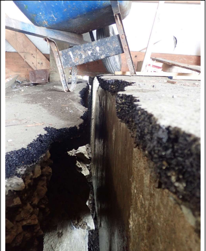
Close-up of settlement and soil failure in Storage Building
