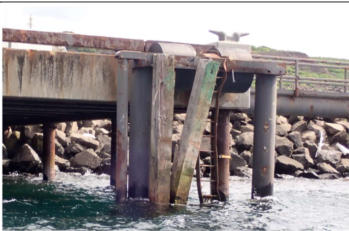
Southern-most fender panel, consider the “lead-in” based on damage. Labelled #1. Impact damage to support piles, only 1 of 8 original fender timbers intact.
