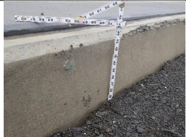
Settlement and Crack Depth at Dock Abutment, Typical
