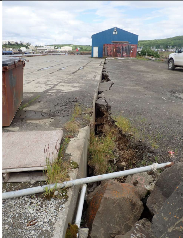
Looking north along soil failure at dock/road interface
