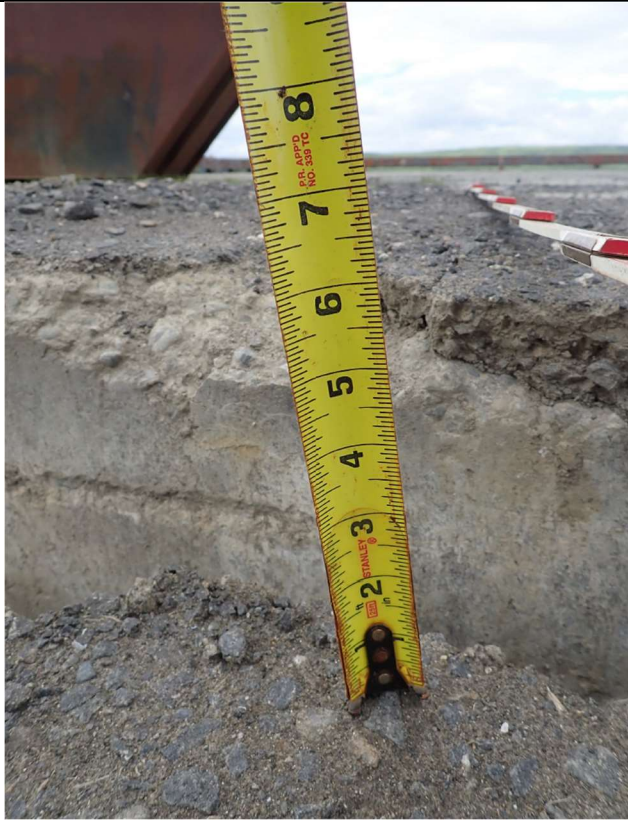
Settlement varies at the Old Dock ~7-8 inches
