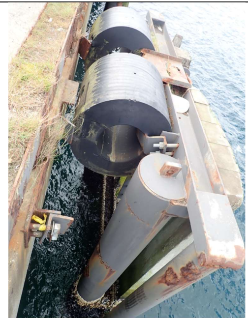
Fender panel #4 is not attached to the dock, and the entire panel is displaced ~33-inches to the south.
