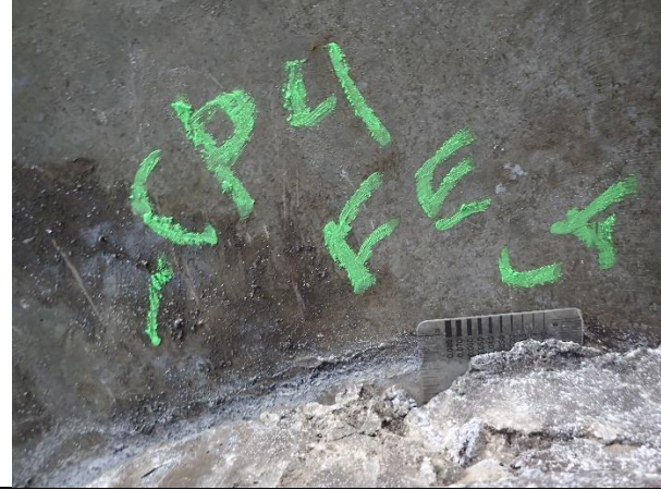
Pile to Pile Cap Interface Crack Penetration, Typical
