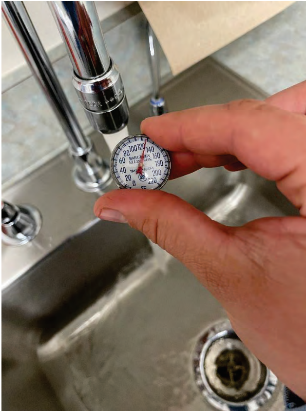
Photo 1: Water above recommended temperature of 120°F.
