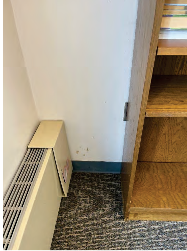
Photo 8: Chipped wall in waiting room.
