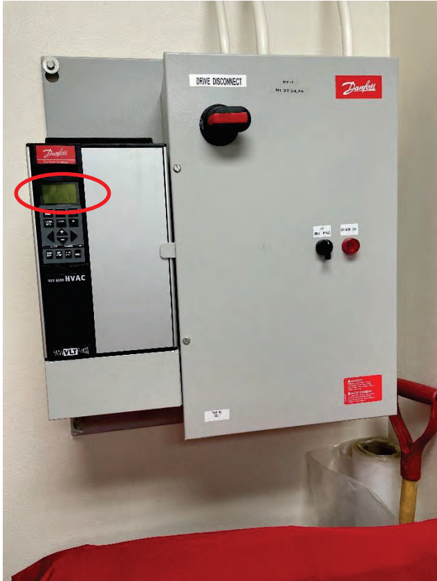
Photo 10: HVAC system screen appeared off.
