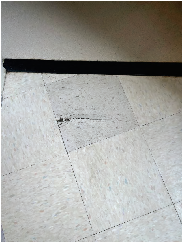
Photo 7: Cracked and chipping tiles were present throughout clinic.
