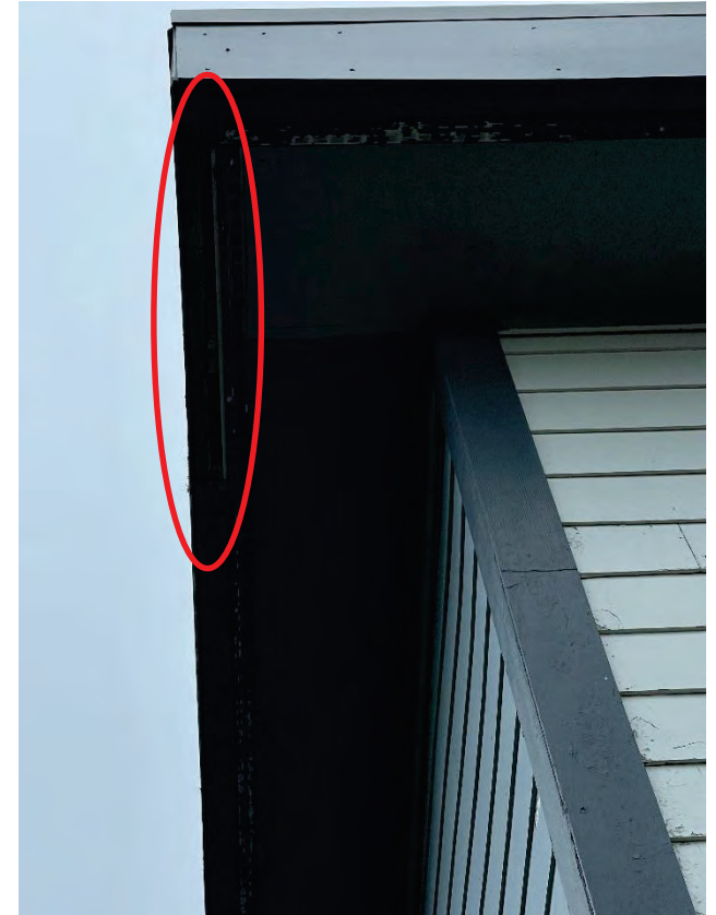
Photo 12: Building roof exterior missing trim.
