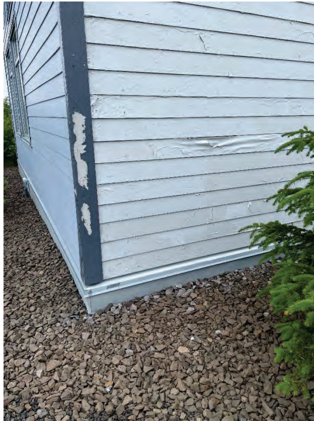
Photo 11: Building exterior paint chipping.
